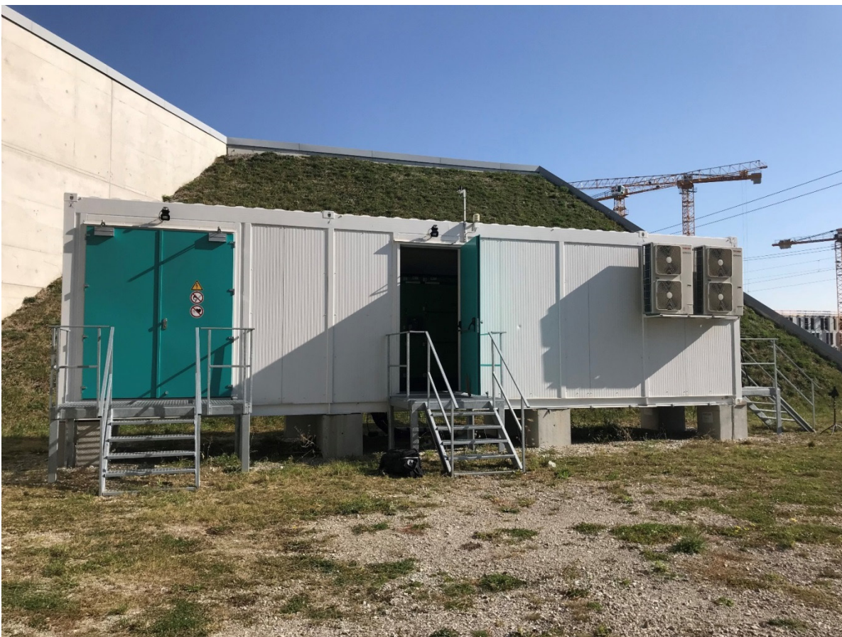
Figure B.1 — Battery storage in Freiham (Image from Stadtwerke München)
